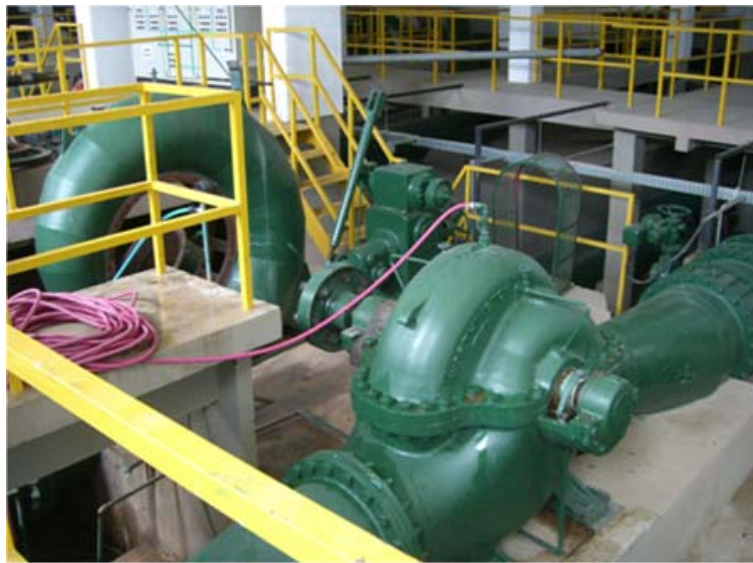
Figure 4. Hydraulic structures i.e. storage tanks, pumping stations, water sources, control valves were properly schematized
