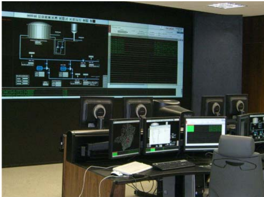
Figure 6. The new telemetry system was installed by Telvent. The link between SCADA and hydraulic mode was developed
